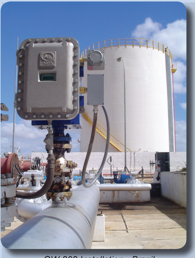
OW-202 Installation - Brazil
