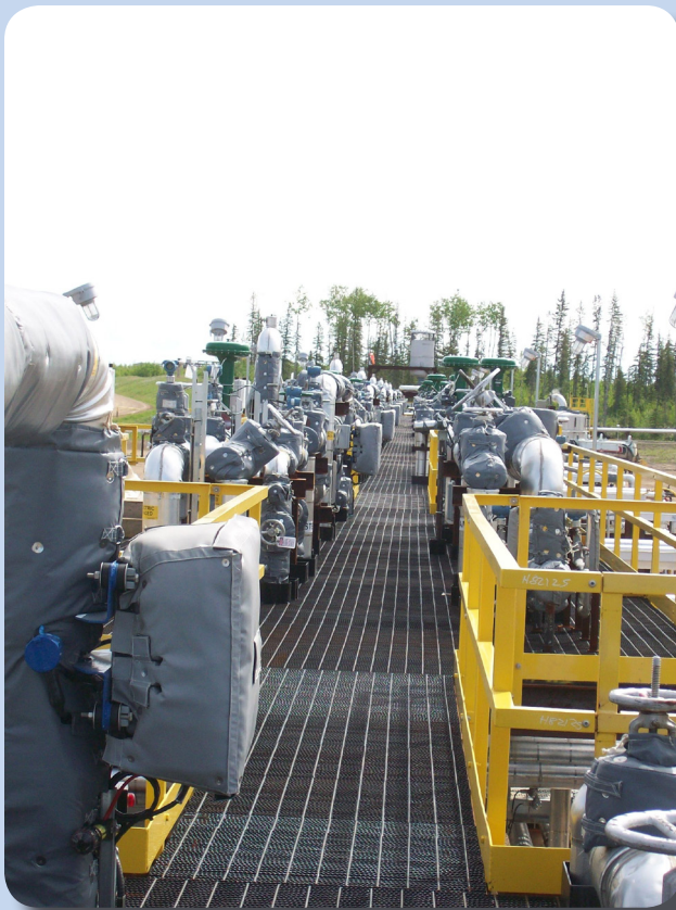
OW-201 Installation - Canada
