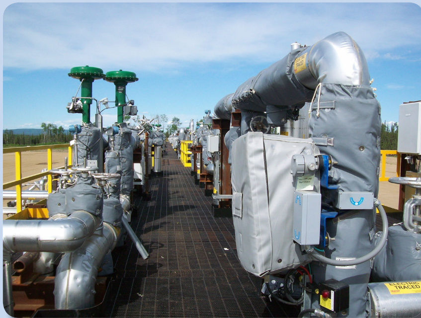
OW-201 Installation - Canada
